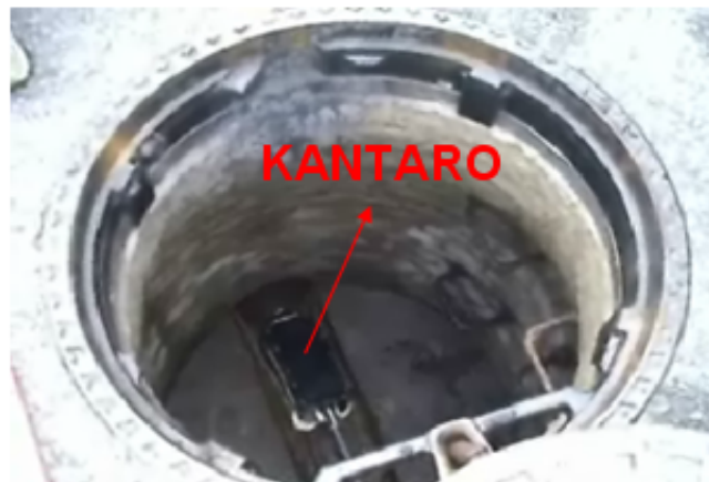
Figure 5.49: KANTARO in real world sewage pipe network while passing a manhole.
