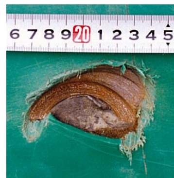
Photo 5 Damage by boring machine
