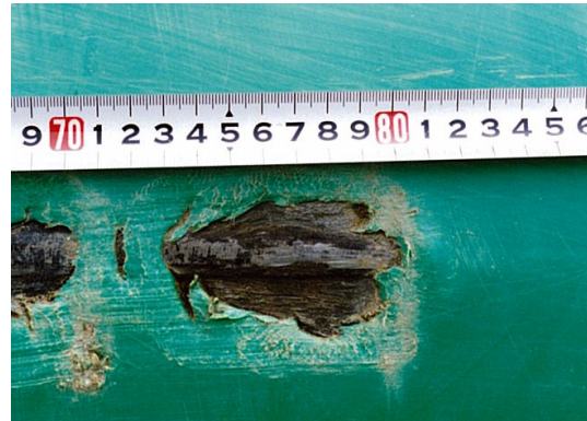
Photo 2 Damage by backhoe
