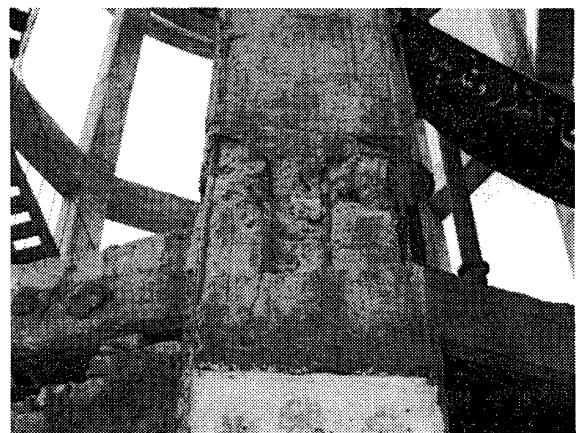
Photo 12 Concrete column and rebar on the east side of the water tank shown in Photo 11
