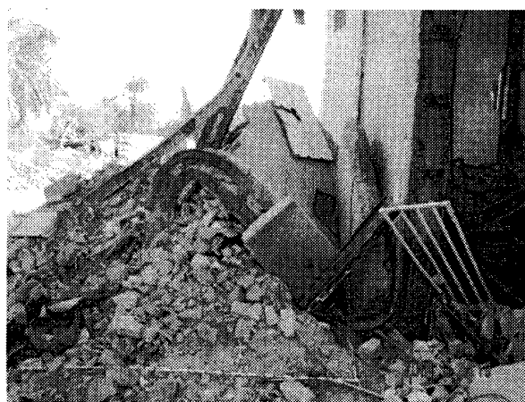
Photo 13 Collapsed steel frame building near by the water tank. This building was dislocated about 1.3 meters westward (rightward)
