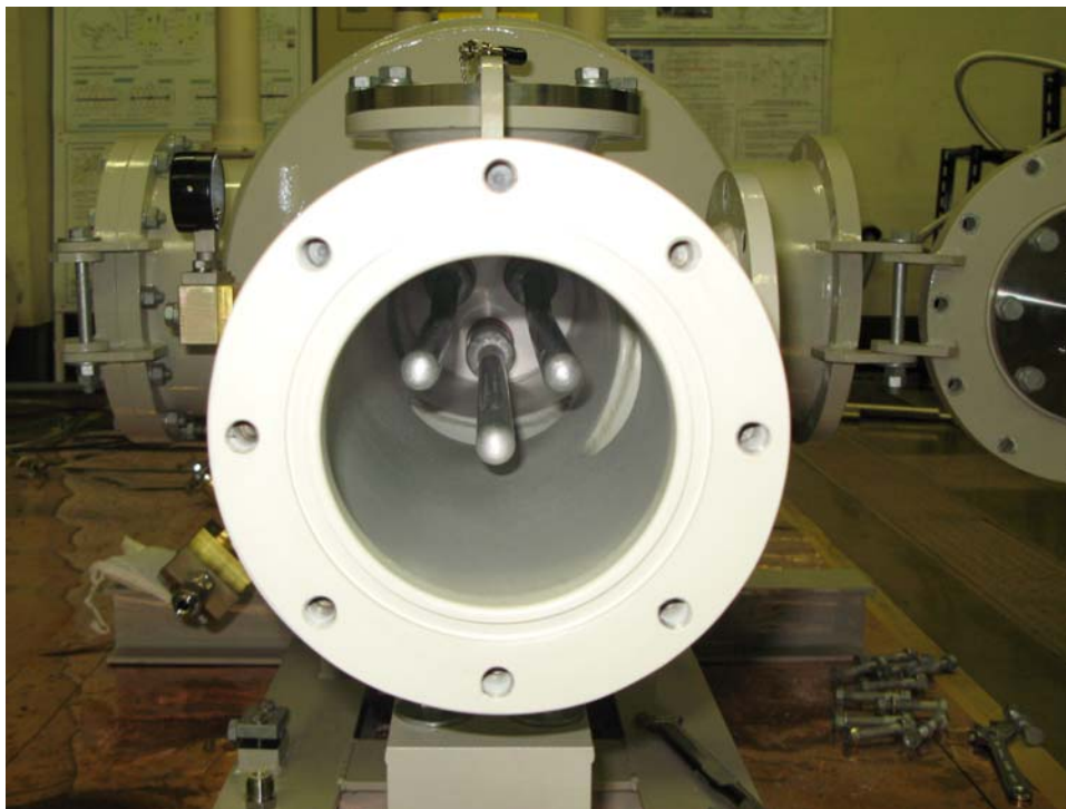
Fig. 2.7 Photograph of three-phase conductors inside GIS model II
