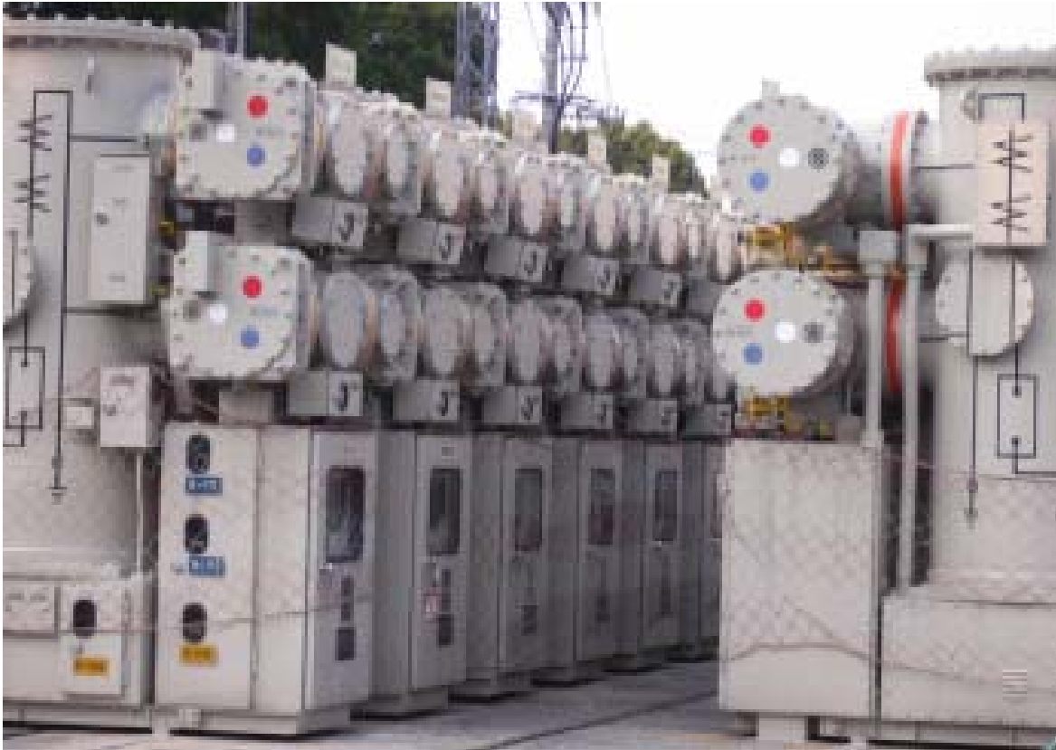
Fig. 1.4 Photograph of three-phase gas-insulated switchgear
